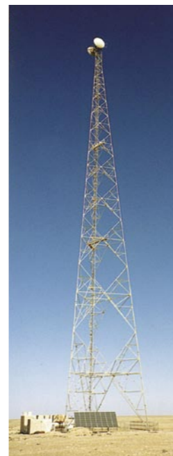
Sollatek has plenty of experience in the telecom field. This project was completed for the Libyan Government in 1998.
