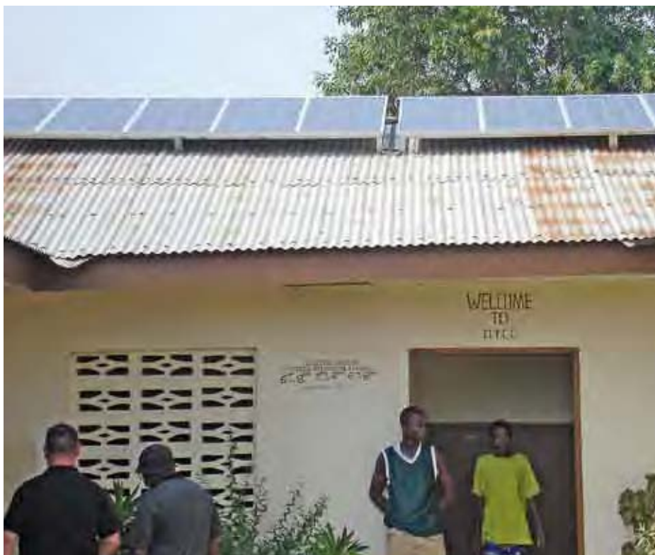
1Kw solar generator - Dolo Town community clinic
