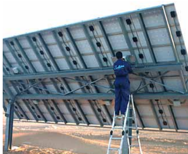
Sollatek technician at an installation site in the Libyan desert
